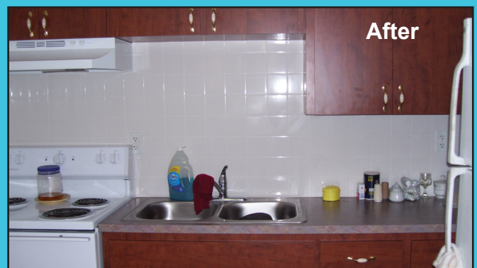
Before and after photos of repairs financed with State Housing Initiatives Partnership (SHIP) program and HOME Investment Partnerships Program (HOME).
